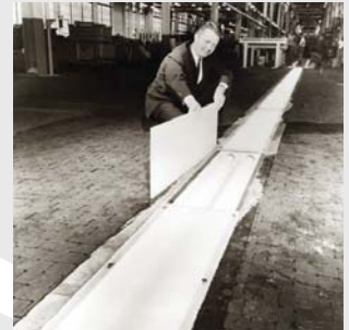
Paramount's In-Floor Pit Lite, a fluorescent fixture installed in the floor of GM assembly plant. This luminaire was rugged enough and strong enough to run lift trucks over.
